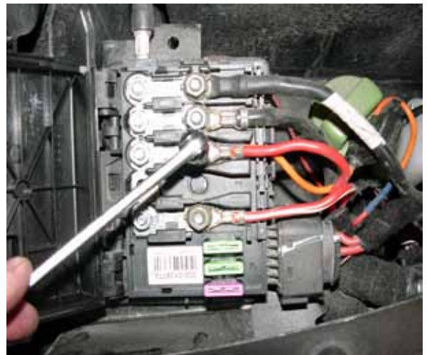
2. Disconnect this cable and protect it from touching other cables around it. Restore cable and cover after the programming.
